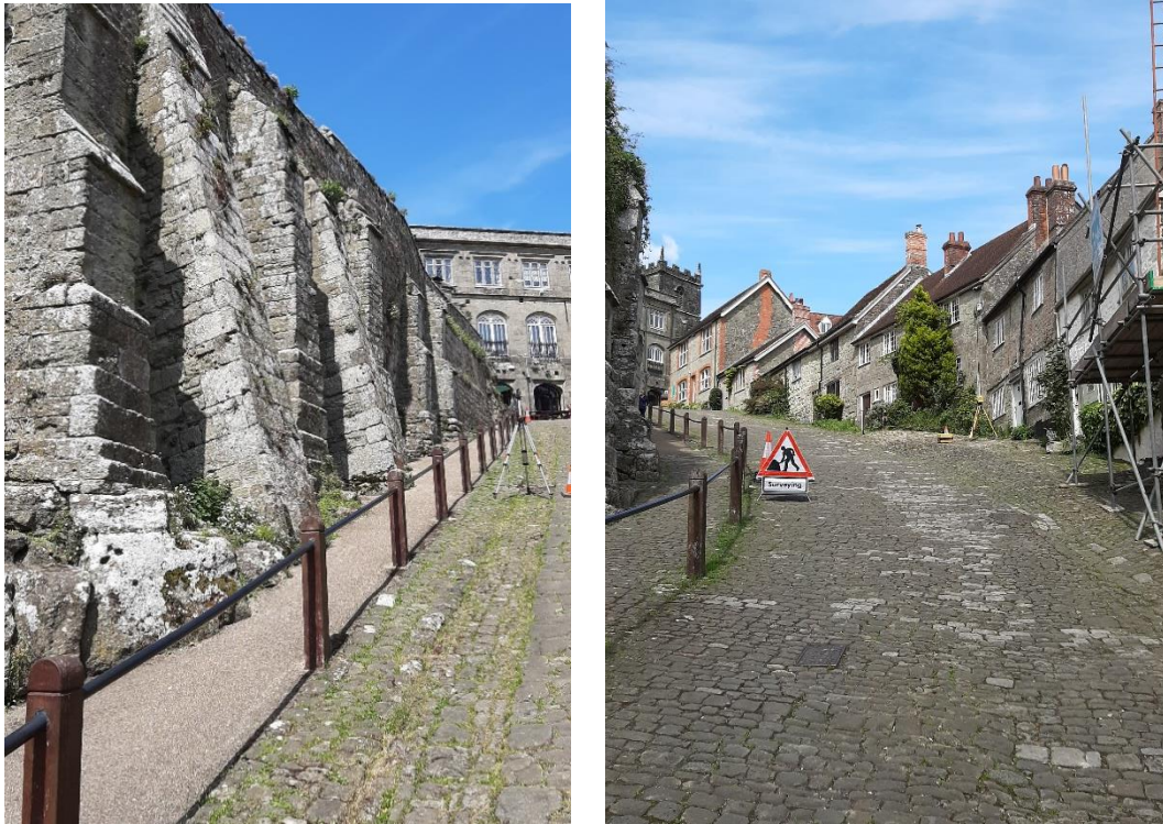
Figures 1 & 2. A section of the scheduled monument and a view of the site at Gold Hill, Shaftesbury. (Author's Image, 2023)
