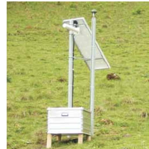
Figure 2b: GNSS SN (Novatel Smart Antenna, WLAN-Antenna, solar panel, alu-box with battery, charge controller and wireless device server).
