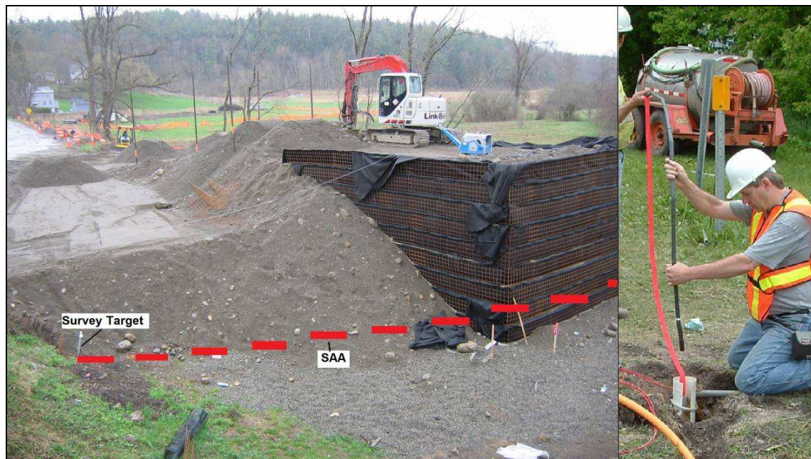
Figure 3 - Left: 2D Deformation Monitoring Near a Bridge Abutment Right: Installation of an SAA for 3D monitoring
